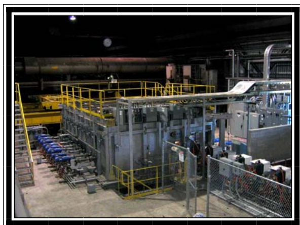
View of the Core holding furnace with the aerial transfer visible in the background.
